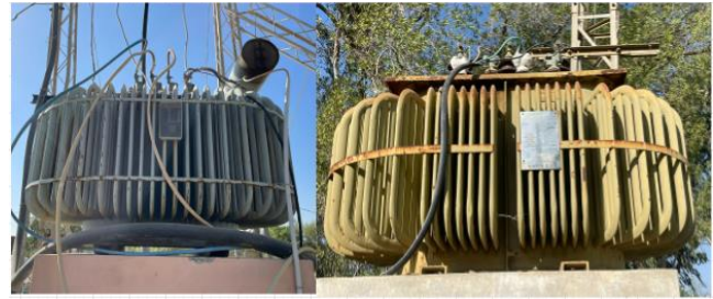
Fig. 3 Figure of Case Study Distribution Transformers A and B
